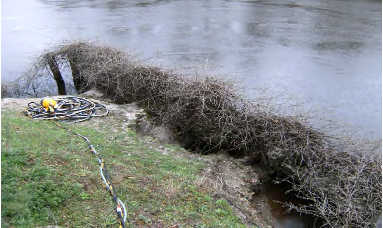
Southern piling bulkhead on east side of river. Note loss of bank behind bulkhead.
