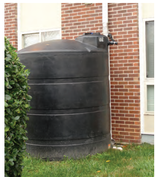
Figure 5.7. Larger above-ground tank made of opaque and durable material.
