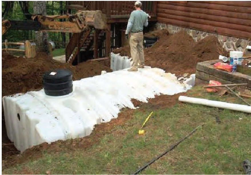
Figure 5.5. A residential system with a large underground tank adds complexity (Source: Rainwater Management Solutions, Inc.)
