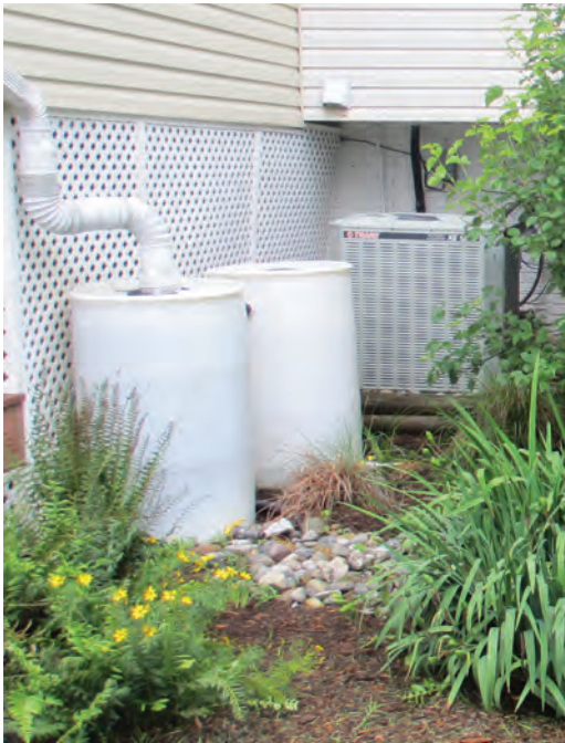
Figure 5.8. Two Rain Barrels connected together to capture more roof runoff
